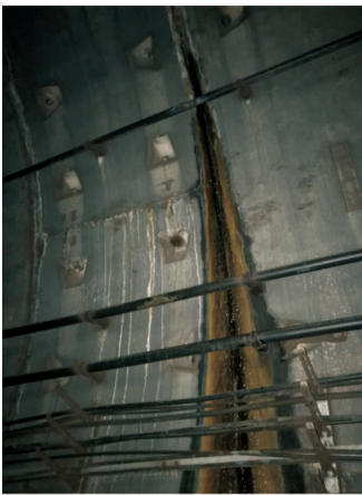
图3 洞门处区间盾构管片接缝渗水 Fig.3 Water leakage at the joint of segments at tunnel portal
