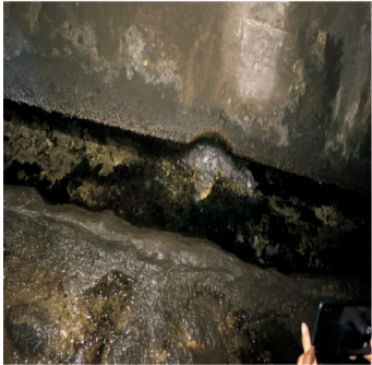
图4 洞门处道床渗水 Fig.4 Water leakage at portal ballast bed
