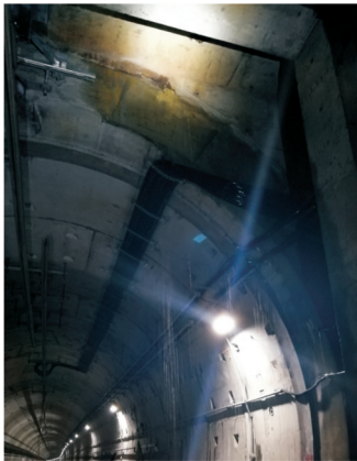
图2 洞门环梁与车站结构内衬墙接缝渗水 Fig.2 Water leakage at the joint between portal ring beam and lining wall
