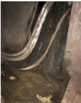
图5 洞门环梁接水槽渗漏水 Fig.5 Water leakage at water catcher of portal ring beam
